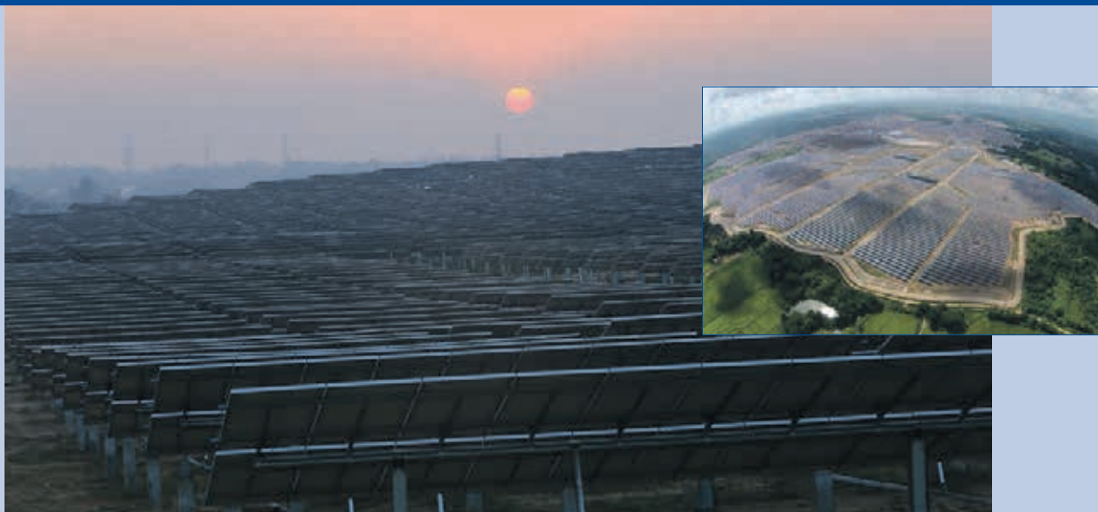
Fig. 3 - The Biggest SPP Project in 2015. This project has achieved COD since February 2015 in Lamphang province. Total installed capacity 126,396 MWp with Poly Crystalline Solar Cell, Solar Tracking System (Photos: Energy Absolute Public Company Limited).
