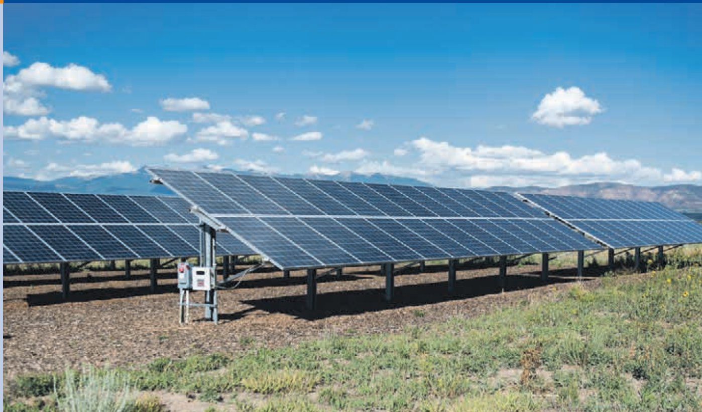
Fig. 3 - A ground mounted PV system in Southwestern Colorado, USA.
