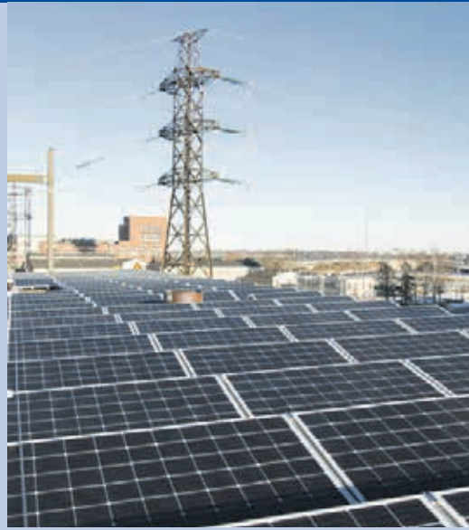
Fig. 2 - Suvilahti Solar PV plant in Helsinki (Photo: Helen Oy www.helen.fi ).
