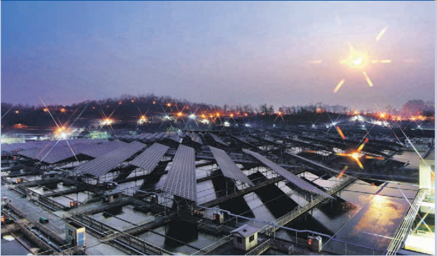
Fig. 3 - 5 MW PV power plant at Amsa Arisu Water Filtration Center, Seoul, Korea (Photo: Hankook-Ilbo).
