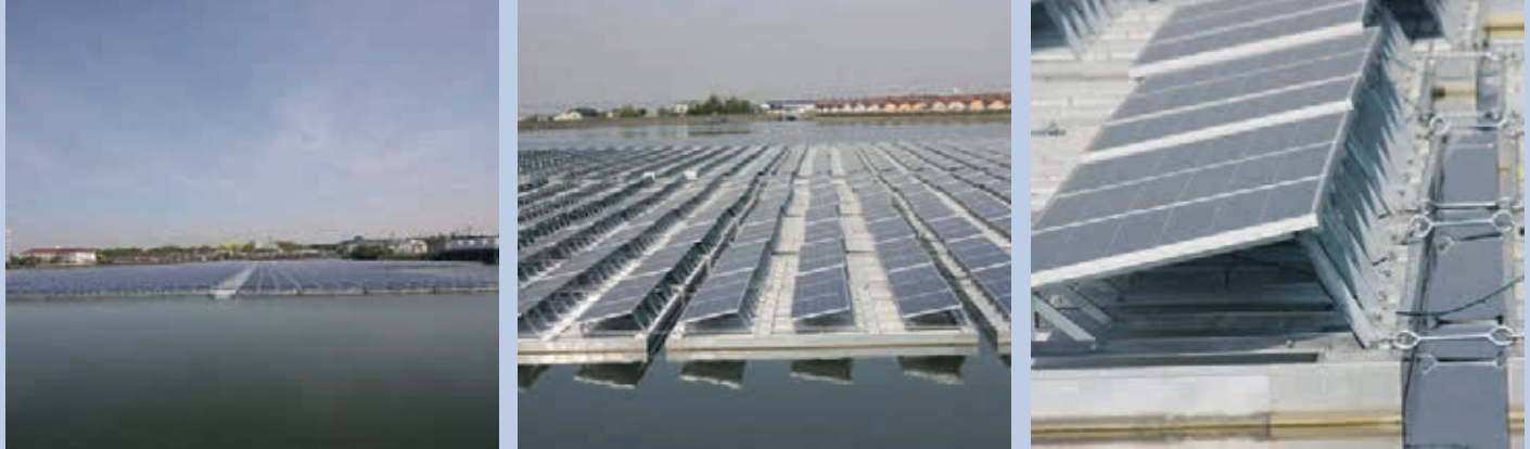
Fig. 1 - Floating PV Power Plant (INFINI Hyogo Daikyū Power Plant) (Inami Town, Hyogo Prefecture). Multicrystalline silicon PV module: 250 W x 6 846 modules (by INFINI) 1,7 MW.
