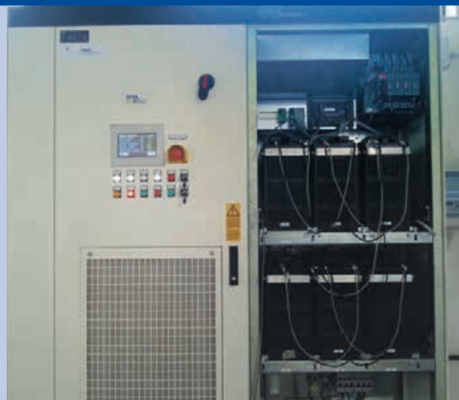
Fig. 3 - Li-Ion Energy storage system (16 kWh) for 14 kWp grid connected PV plant on Lampedusa island (Photo: ENEA, www.enea.it ).
