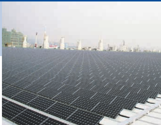
Fig. 2 - 3 MW roof mounted PV system at LG Electronics, Gumi-si, Gyunsangbuk-do, Korea (Photo: Solar Today).
