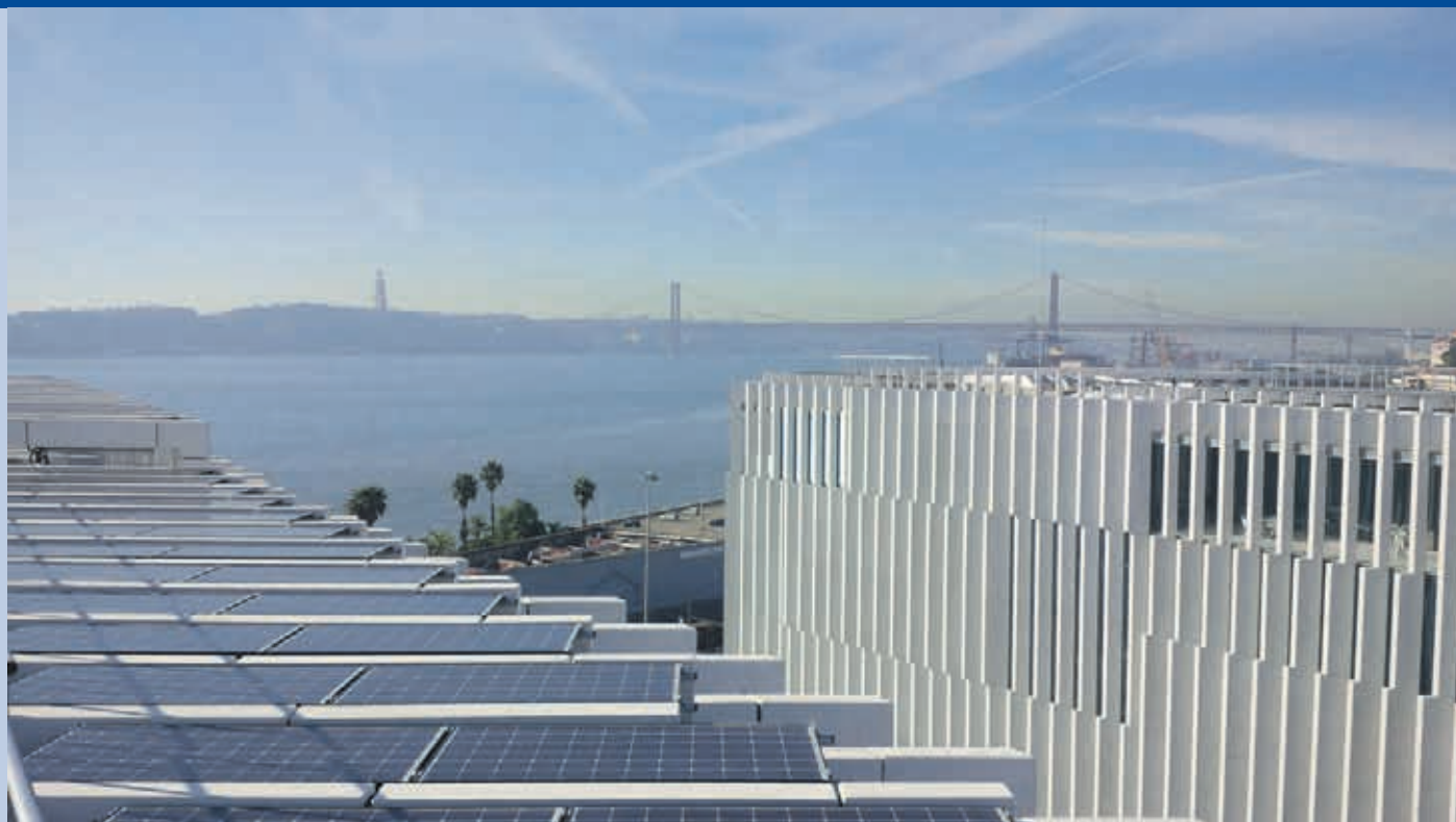
Fig. 1 – New EDP Headquarters in Lisbon – 84 kW PV self-consumption.
