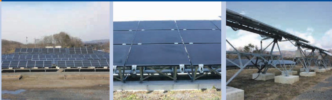
Fig. 3 - Fukushima Airport Mega-Solar Power Plant (Sukagawa City, Fukushima Prefecture, etc.). Total: 1,2 MW (500 kW, 200 kW, 500 kW), 30 types of PV modules including tracking system and various types of mounting structures.
