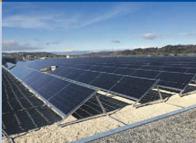
Fig. 2 - Self-consumption 658 kW PV system on a MIGROS supermarket with bifacial glass-glass modules, Schönbühl (Photo: Genossenschaft Migros Aare).
