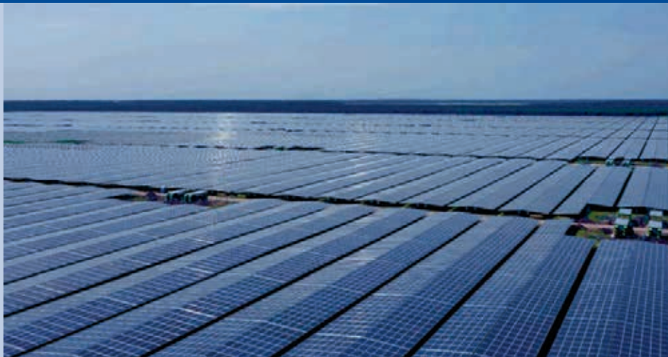
Fig. 3 – 230 MW PV plant, near Bordeaux, mounted on fixed structures with an east-west orientation (Photo: Neoen, Clemessy).
