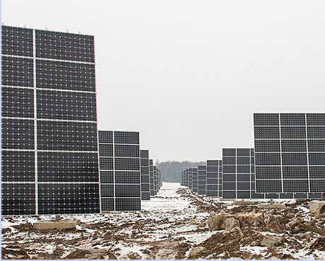
Fig. 1- The first Swedish MW-installation was constructed during 2013. Solar trackers are rather untypical for Sweden, and the site is participating in a monitoring study (Photo: Bengt Stridh, ABB/Mälardalens högskola).
