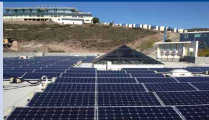
Fig. 2 - 75 kWp Grid Connected PV System at CICESE Ensenada Baja California, Mexico (Photo: Solartec).
