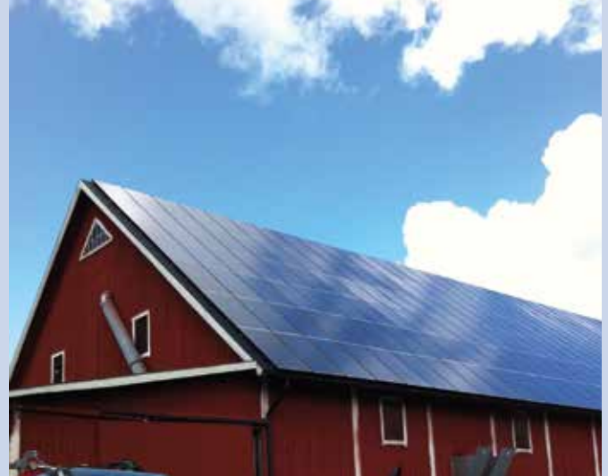
Fig. 2 - Solar panels on barn roof (Photo: PPAM.se Sweden AB).
