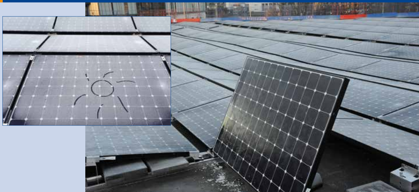
Fig. 4 - PV installation at Powerhouse Kjørbo, delivered by Direct Energy. The system has a capacity of 310 kWp (See also www.powerhouse.no ).
