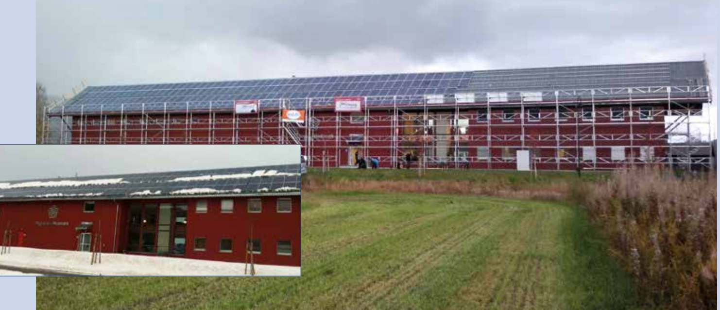
Fig. 1 and 2 - PV installation at Høgskolen i Hedmark, Avdeling Evenstad. 70 kWp system supplied by FusEn AS.
