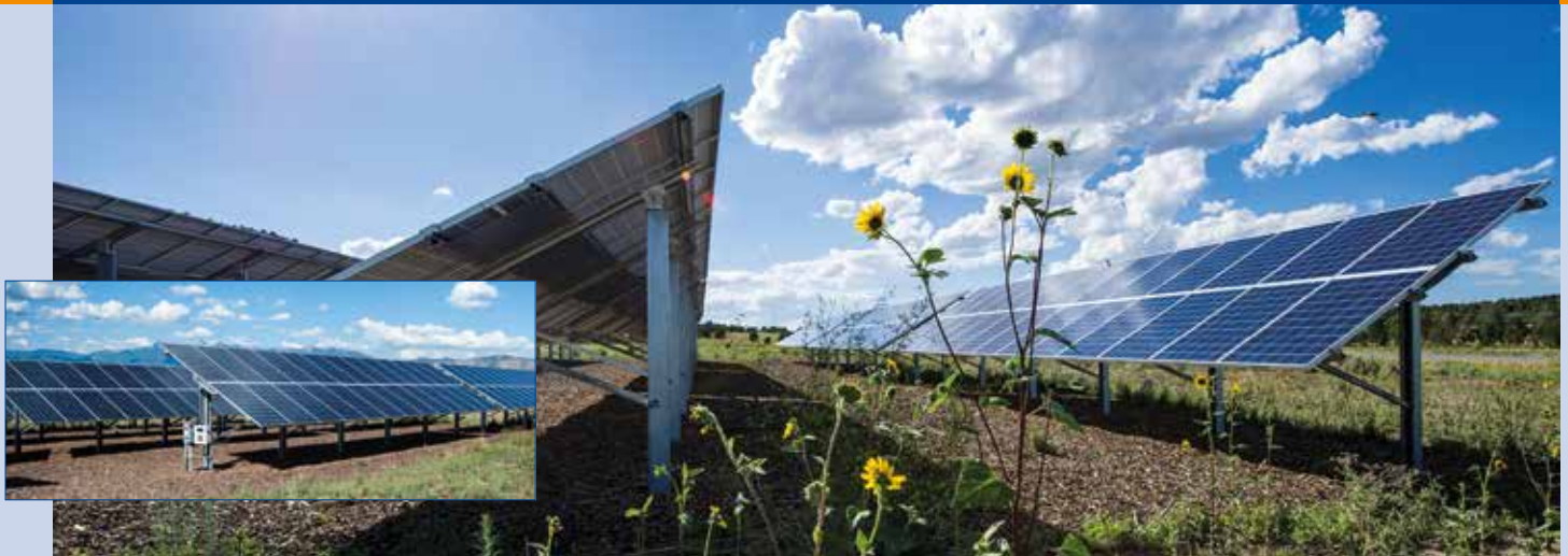
Fig. 3 - 67 kW (STC rating) photovoltaic array at the Mesa Verde Visitor and Research Center in Montezuma County, Colorado. The array consists of 286 Schott Poly 235 watt solar modules (13,8 % efficiency) wired in 22 series strings of 13 modules per string. Coupled with a micro-hydro system and solar water heating, the on-site renewable energy systems are capable of providing 95 % of the building energy requirements (Photo: Dennis Schroeder / NREL).
