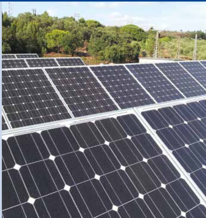
Fig. 1 - 5 kWp residential microgeneration project.
