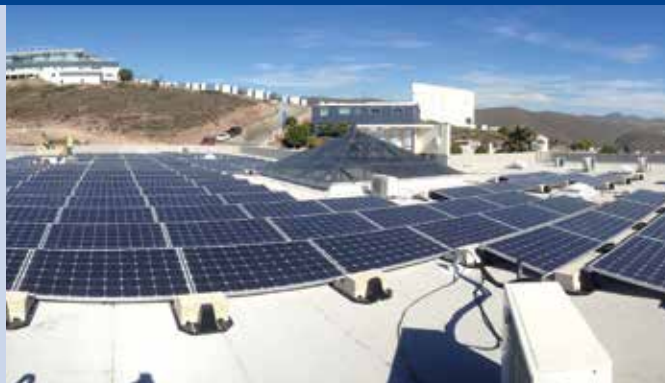
Fig. 1 - 75 kWp Grid Connected PV System at CICESE Ensenada Baja California, Mexico (Photo: Solartec).
