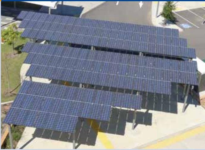
Fig. 2 - Shade shelter at bus and taxi rank, Townsville RSL Stadium. The 20 kW array (153 x Kyocera KD135W modules) is part of the Townsville Queensland Solar City Project (Photo: Ergon Energy).
