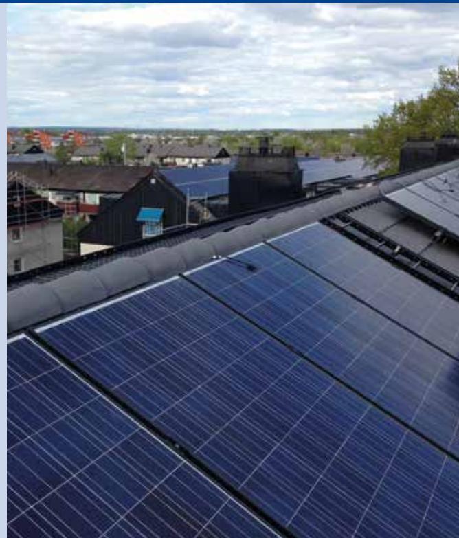
Fig. 4 - PV modules on several apartment buildings. 624 kW in total (Photo PPAM.se Sweden AB).
