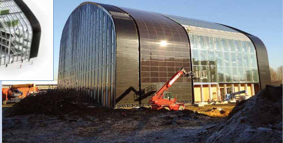
Fig. 1a & Fig. 1b - Bruxelles Environnement. The new Brussels Environment and Energy Administration Headquarters will be the largest passive office building in Europe and will include 700 m 2 of BIPV ISSOL modules (Photos: Copyright CEPEZED, ISSOL for Fig. 1a and ISSOL for Fig. 1b).
