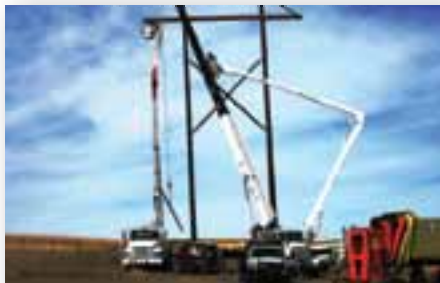
4MW Ontario Energy Storage Project
