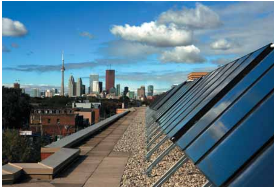
Mondial Energy’s 108 panel solar thermal system for Woodgreen Community Services in Toronto. Photo courtesy of Mondial Energy.
