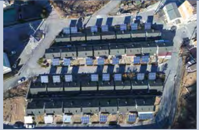
Fig. 2 - Combined PV and solar thermal system, Samcheok-si, Gangwon-do, Korea.
