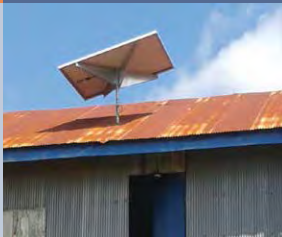
Fig. 6 - Solar panel on residential house, Cambodia, 2017 (Photo: IED, France).
