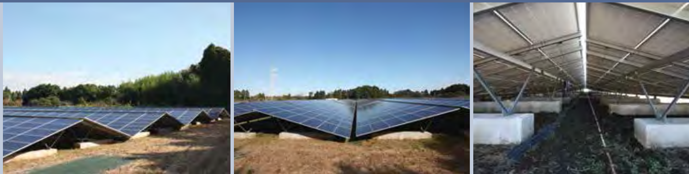
Fig. 1 - Ground-mounted PV System arranged in the east-west direction with an M shape (F Nagara PV Power Plant) (Nagara-machi, Chosei-gun, Chiba Prefecture). 1,905. 1 kW Multicrystalline silicon PV module (by Suntech) (315 W).
