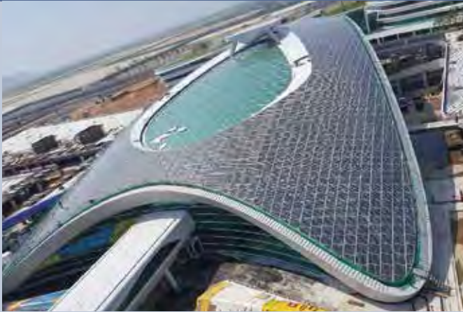
Fig. 1 - 1 638,48 kW PV system installed at Incheon Airport Terminal 2, Incheon, Korea.
