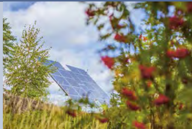
Fig. 2 - LUT two-axis solar PV tracker (Photo: Lappeenranta University of Technology).
