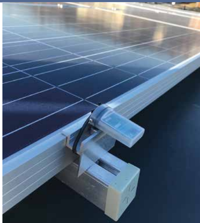
Fig.1 - PV system at Uppsala Science Park used in the UppScaleSolar project with the sensor for solar irradiance measurement (Photo: Joakim Munkhammar).
