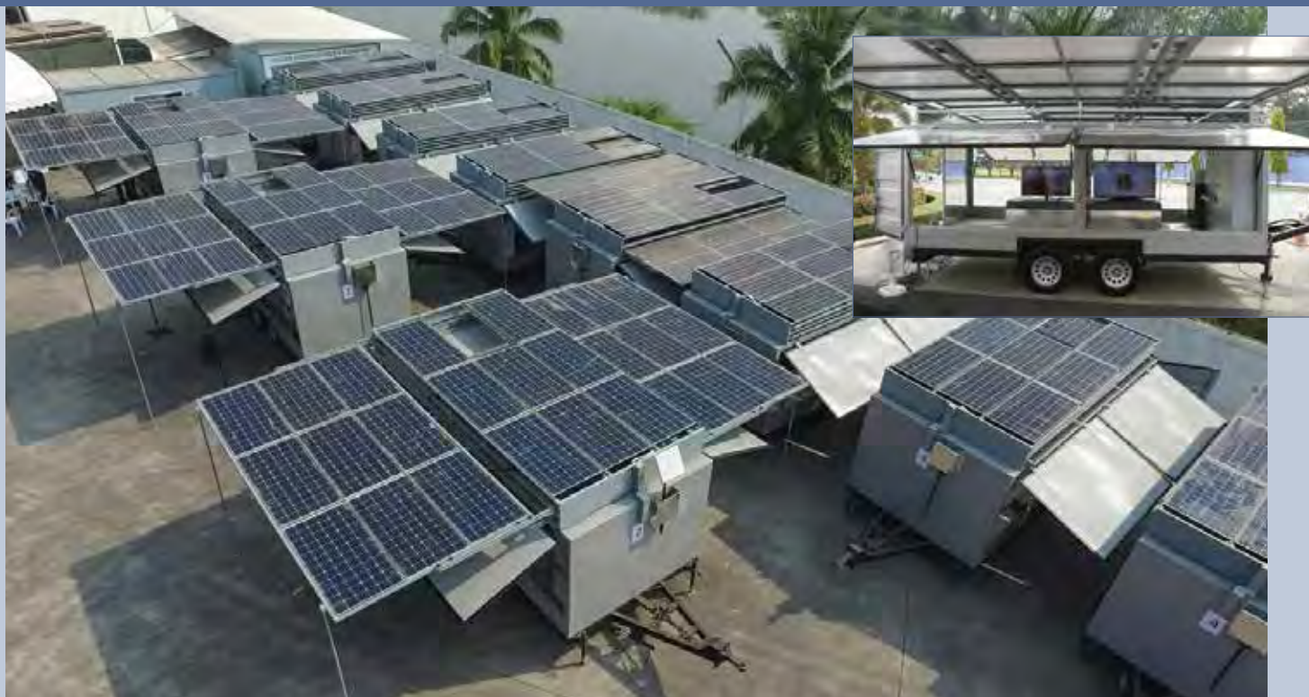
Fig. 1 – The Mobile Solar Cells Trailer Project to Support Electric Power in Three Southern Border Provinces for Military Units and Neighborhoods. Capacity of 6 kW / vehicle, a total of 12 vehicles can replace about 130,000 units of electricity per year, operated by the Internal Security Operations Command and support budget by the energy conservation fund (Photo: DEDE).
