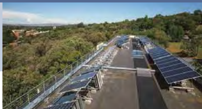
Fig. 2 - CSIR outdoor PV testing facility installed on the roof of the Energy Centre on the CSIR campus in Pretoria.
