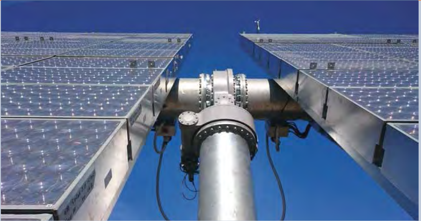
Fig. 3 - CPV plant installed at Monteveglio (BO) in the frame of the EU funded Ecosole project (Photo: Beghelli Becar).
