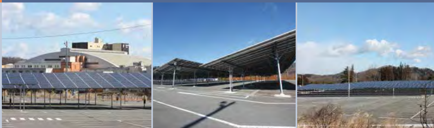
Fig. 3 - PV System for a Parking Lot (Spa Resort Hawaiians) (Iwaki City, Fukushima Prefecture). 2.1 MW Multicrystalline silicon PV module (by Yingli, 275 W x 7,627 modules).
