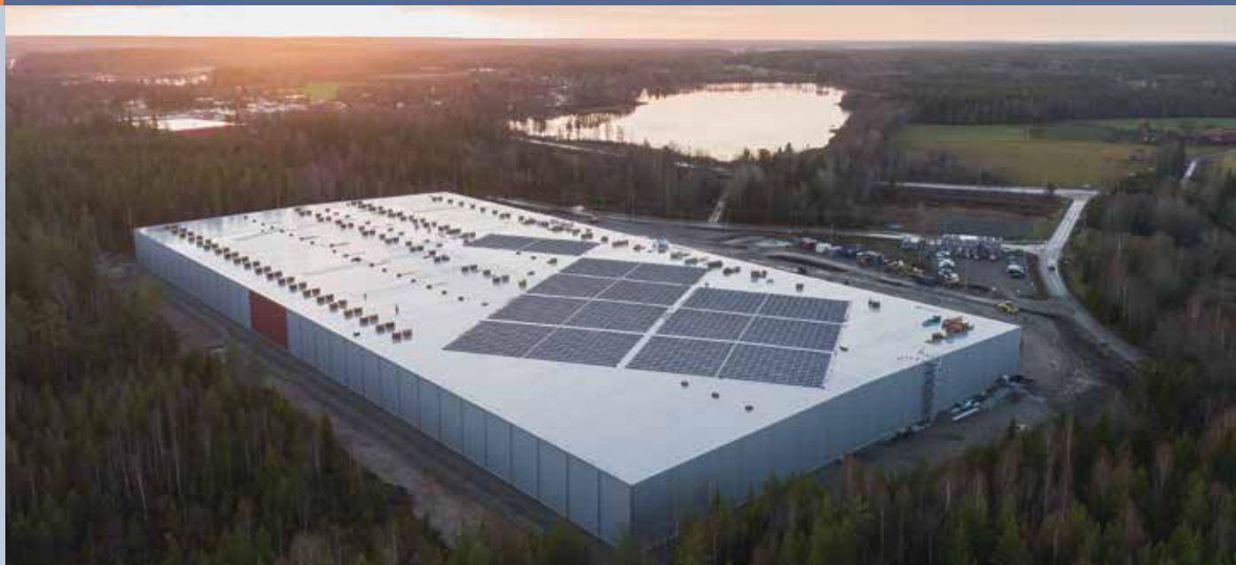
Fig. 2 - Apotea's warehouse and logistic center in Morgongåva - 1 500 kW - Sweden's largest roof-mounted PV system (under installation) (Photo: Gustaf Kumlin / Apotea.se).
