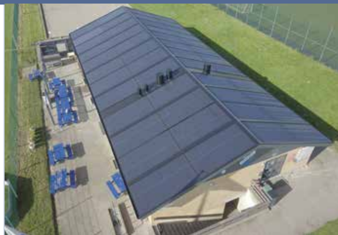
Fig. 1 - PV/T Energy Day at Stenløse Football Club: The innovative "Hercules energy roof" with efficiency exceeding 50 %, was developed and produced by RACELL A/S for the Stenløse club building. The old worn-out and leaking roof was replaced by the new water-tight solar roof. The 7,5 m 2 self-bearing light-weight Hercules modules were fixed directly on-top of the wooden battens, thus the installation took 2 days only. The hybrid PVT roof has a capacity of 520 W/m 2 (electricity 180 W p /m 2 and heat energy 340 W p /m 2 ). The total south roof area is 180 m 2 . The project was supported by the Danish Energy Agency EUDP (Photo: RACELL).
