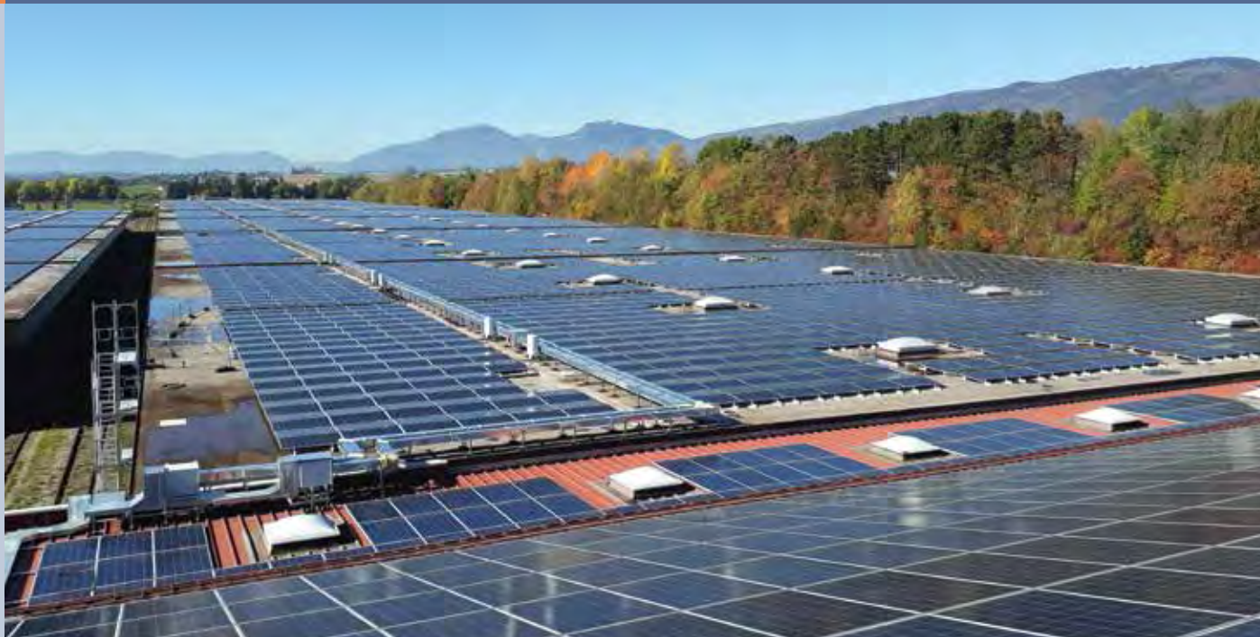
Fig. 3 - PV System at Philip Morris in Onnens, Switzerland. The entire system (mounted on several roofs) is presently the largest PV installation in Switzerland; with a capacity of 8,3 MWp, it produces approximately 8 GWh of solar power per year (Photo: © aventron AG).
