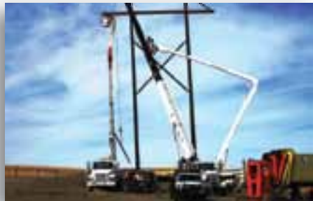
4MW Ontario Energy Storage Project
