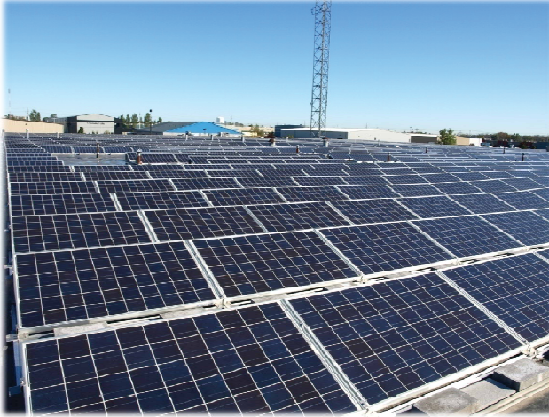
250kW Ballasted Installation PLP Canada – Cambridge, ONT Installed – Summer 2010
