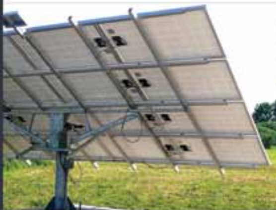
PRM TOP OF POLE
