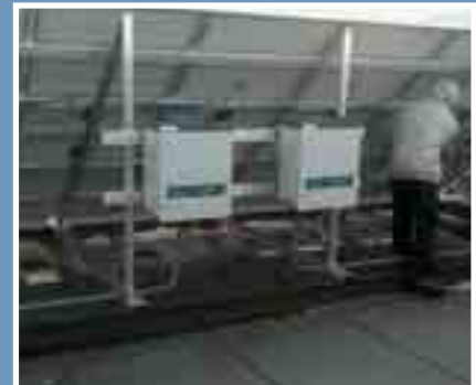
Inverters on a 30kW rooftop system, Medicine Hat, Alberta
