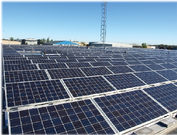
250kW Ballasted Installation PLP Canada – Cambridge, ONT Installed – Summer 2010
