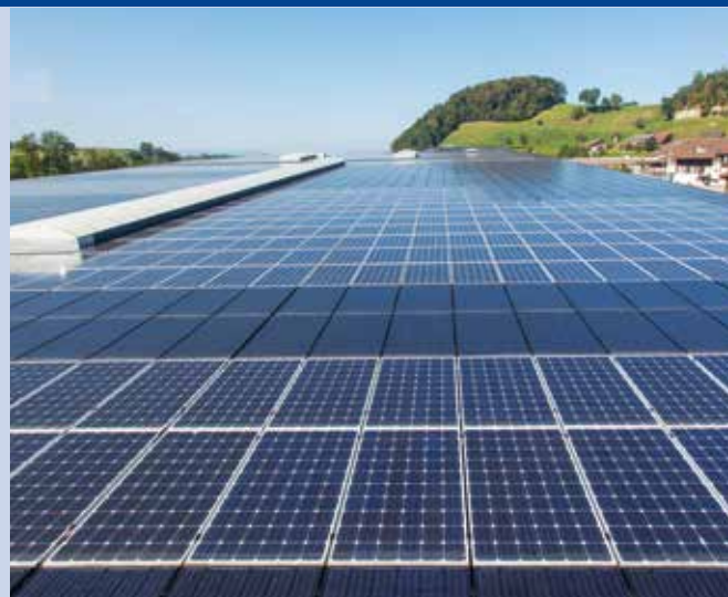
Fig. 3 - 538 kW roof-integrated PV system, Affentranger Bau AG, Altbüren (Photo: © NET Ltd. /DanielForster.com).
