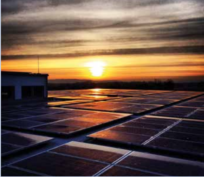
Fig. 1 - Sunrise over 150 kWp installation in Vänersborg (Photo: Solkompaniet AB).
