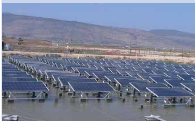
Fig. 3 - Solaris Synergy's solar PV field installation on a water reservoir.
