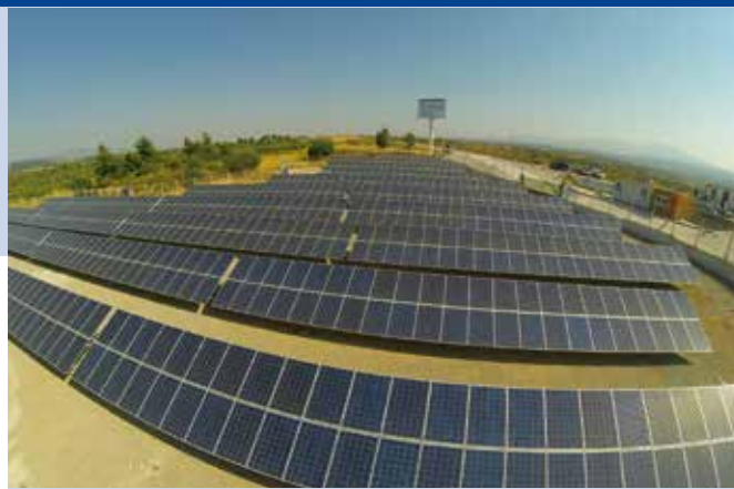
Fig. 2 - 500 kW PV system in Izmir, Turkey; one of the supported projects by IZKA.
