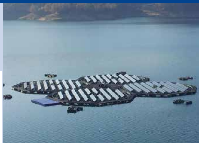
Fig. 3 - 100 kW tracking-type PV power plant on the water surface at Hapcheon Dam, Hapcheon-gun, Gyeongsangnam-do, Korea.
