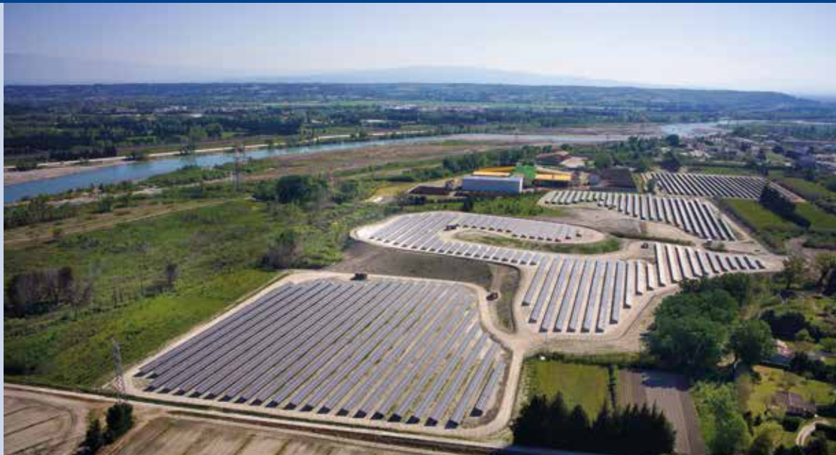
Fig. 3 – Photovoltaic power plant built on brownfields, 7 MW, Chateaufort (Bouche-du-Rhône Dpt), La Compagnie du Vent/ Mydrone.fr (Photo: Lionel Barbe).
