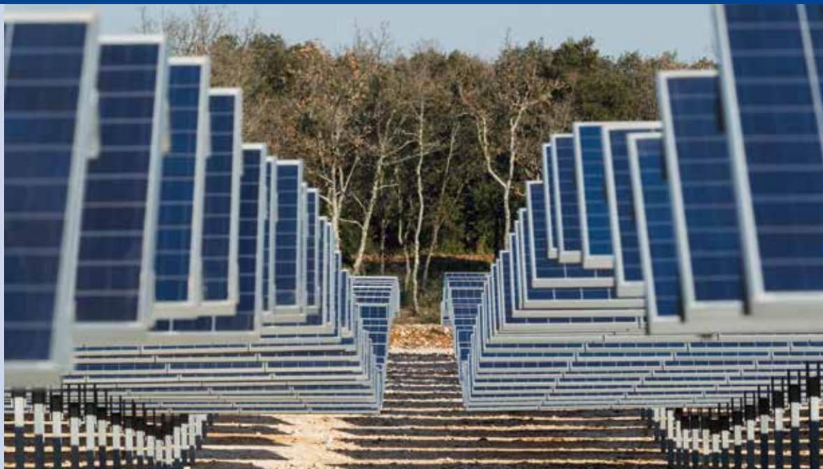
Fig. 2 – Photovoltaic power plant with horizontal single-axis tracker, 4,7 MW, Vallérgues (Gard Dpt), Urbasolar/Exosun (Photo: Christophe Ruiz).
