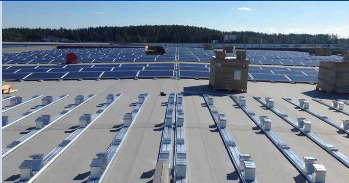
Fig. 1 - At Asko Vestby, a 370 kWp system was installed during the summer of 2014. This is the largest system in Norway, and the system is built solely for self-consumption. The power is delivered to a refrigerated storage (Photo: Multiconsult).
