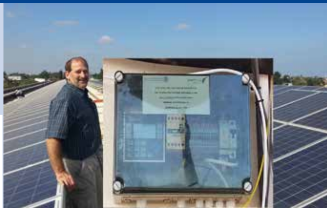
Fig. 1 - MG Lightning monitoring system at a solar PV installation.
