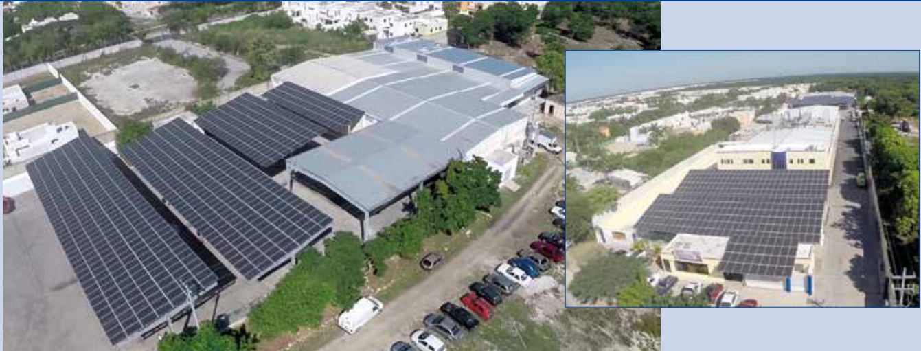
Fig. 1 - 324 kWp PV system installed in the parking lot of a snack factory in Merida Yucatan (Photo: CONERMEX).
