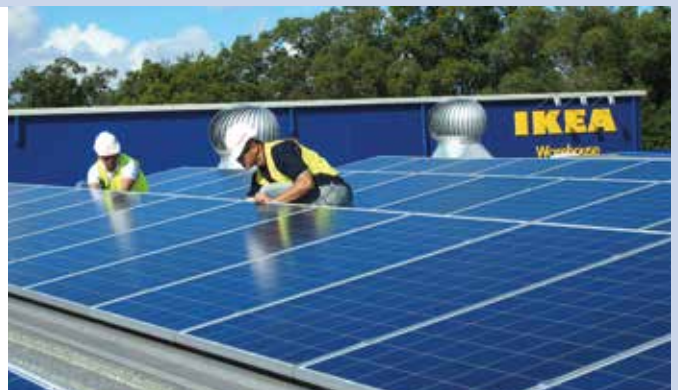
Fig. 2 – IKEA's 3,6 MW Commercial PV Roll-out in Rhodes, NSW (Photo: Canadian Solar, Australia).
