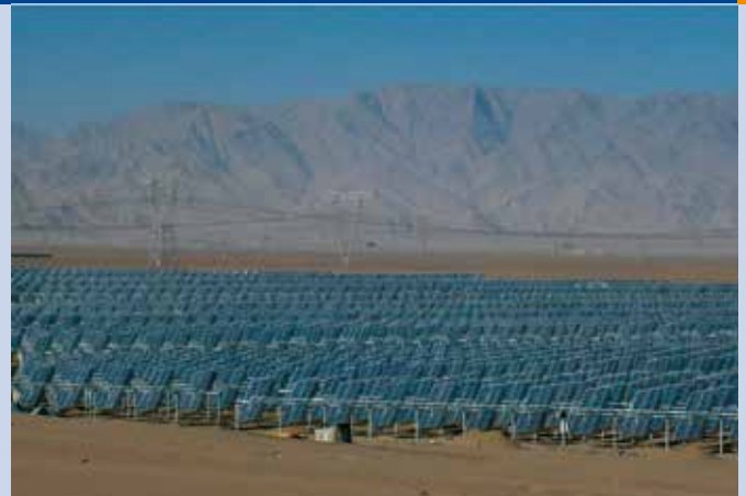
Fig. 4 – Shengguang high concentrating PV (HCPV) power station, Golmud, Qinghai, China.
