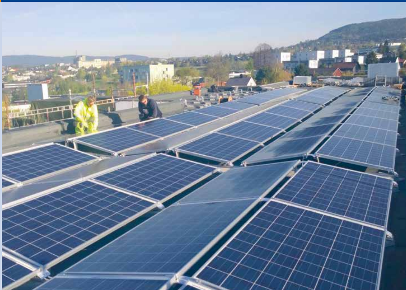
Fig. 2 - Omsorgsbygg Oslo installed a 130 kWp system at Økern Sykehjem (a home for elderly people). The power from the system is for self-consumption (Photo: Fusen AS).
