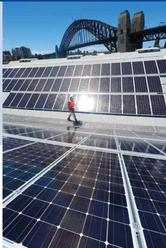
Fig. 4 - Sydney Theatre Company rooftop system (Photo: SF-Suntech).
