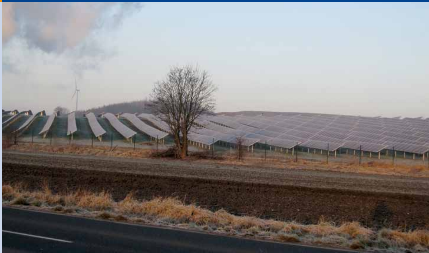
Fig. 2 - Ground mounted photovoltaic installation with 3,9 MW peak power on a former landfill site (Photo: Klaus Prume).
